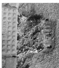
Above: Blocked drains, Station Road
