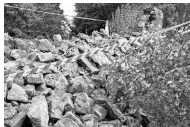
Part of the collapsed churchyard boundary wall
