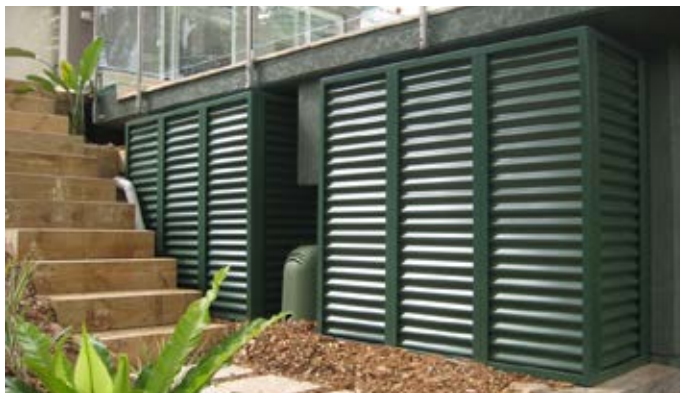
Figure 58: An example of concealed tanks used for rainwater harvesting.
