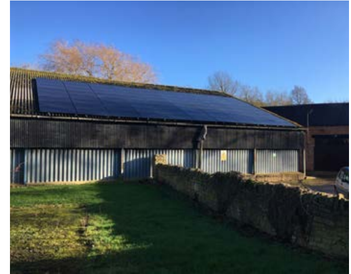
Figure 55: Solar panels on barn in Hargrave.
