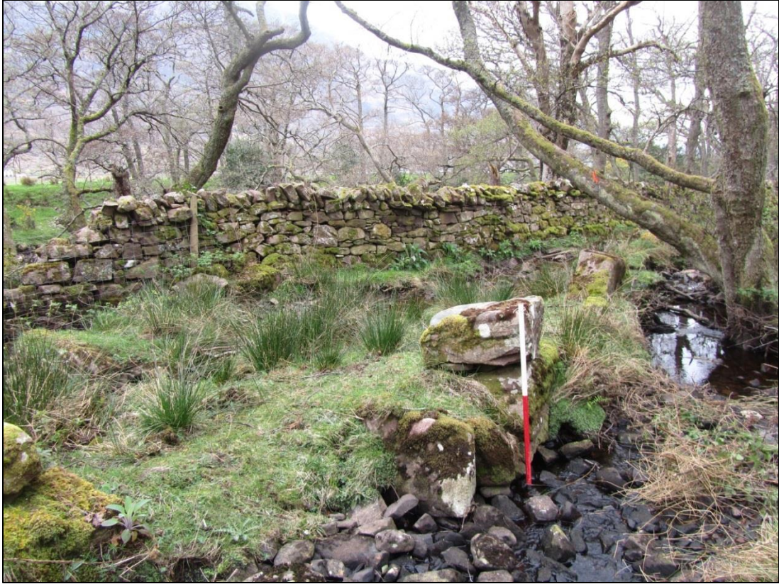
Figure 5: NE corner of Building 13 showing inundation by the burn also wall 35 which cuts through the building
