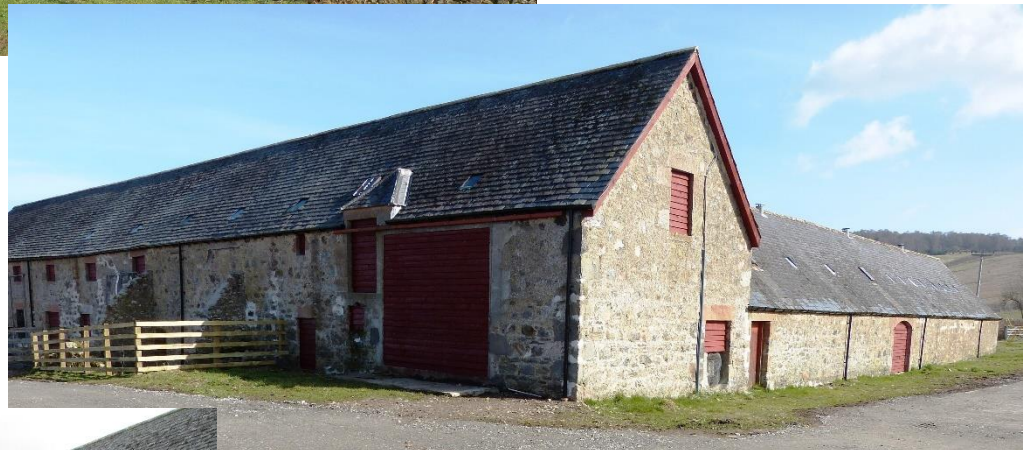
Figure 14: The S corner, With the stables on the right, and north wing on the left © Alasdair Cameron
