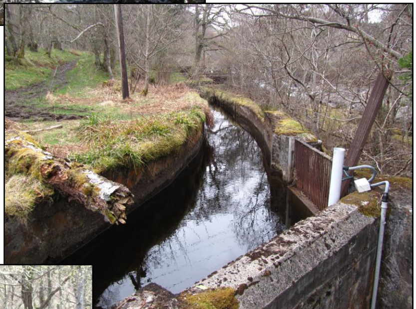
The lade (right) viewed from the east and (below) the west sluice with metal grid and overhead hoist
