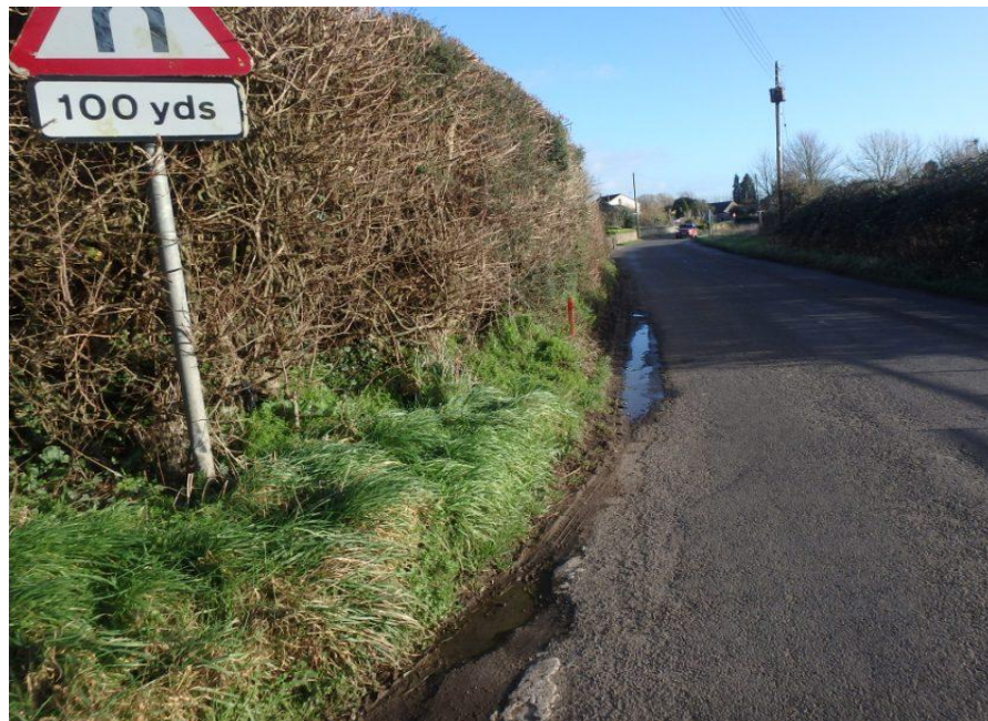
Erosion of grass verge in WR at junction with Bourton Lane
