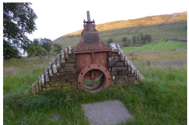
An old Water Shut-off Valve
