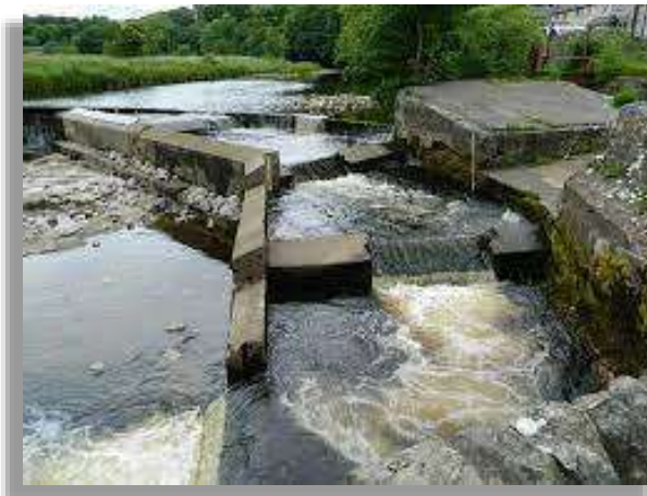
The Fish Ladder part of the Hydro Scheme on the River Ribble at Settle
