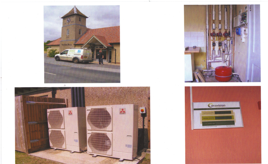
Air source heat pumps installed in August
